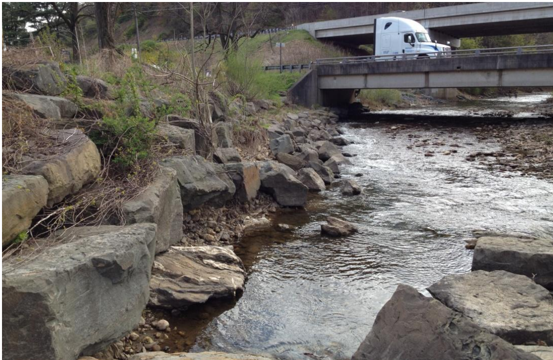
Figure 6 – Image of a failed section of the riprapped bank downstream of the Old Route 15 Bridge (facing upstream).
