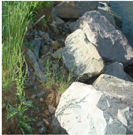
Figure 43 – Image of the bank erosion downstream of the downstream restoration structure (facing upstream).
