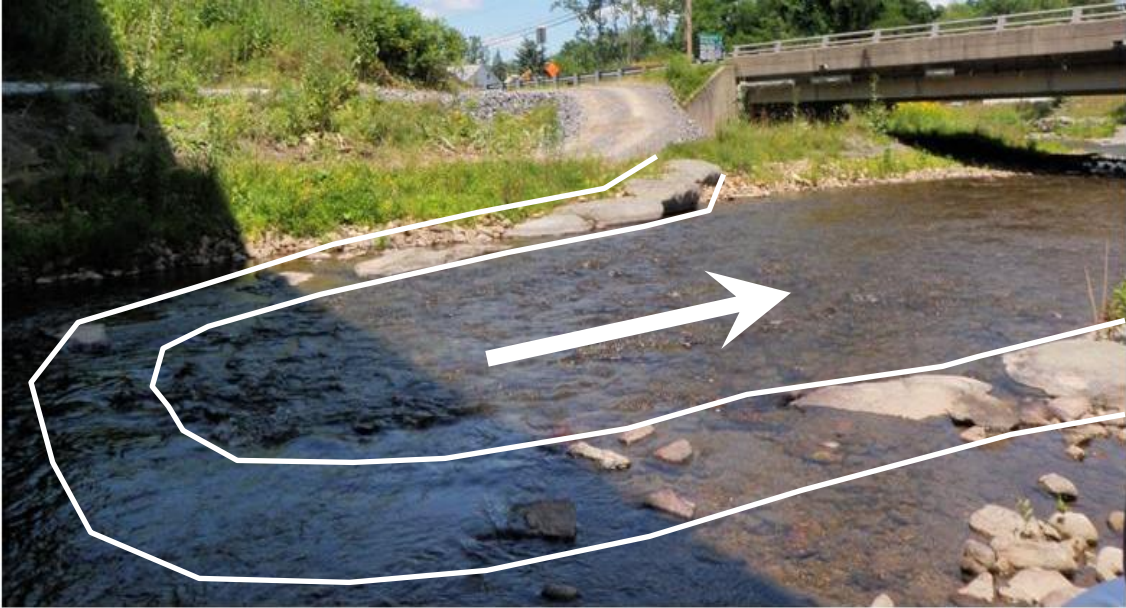
Figure 5 – Image of the upstream rock cross vane (white lines) and the large gravel/cobble sized sediment that has buried it (White arrow shows flow direction).
