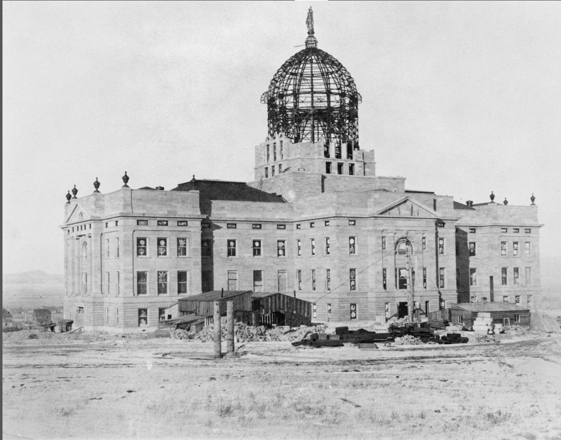
Construction of the dome. Catalog #952-636. ca. 1901. Montana Historical Society Research Center Photo Archives. Helena, Montana.
