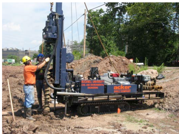
Figure 7. Photograph of BU track-mounted drilling rig at SB cutoff wall field site in Birdsboro, PA (2009).
