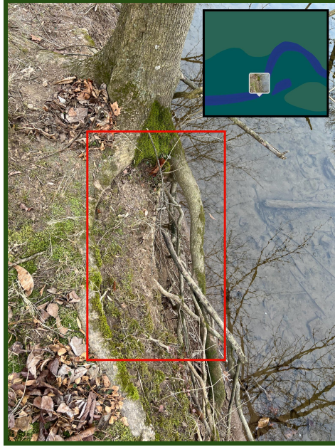
Figure 5: Example of bank erosion along the lower portion of Dale’s Ridge Trail that borders Buffalo Creek. Exposed roots are highlighted in the boxed area. (Map from iPhone)
