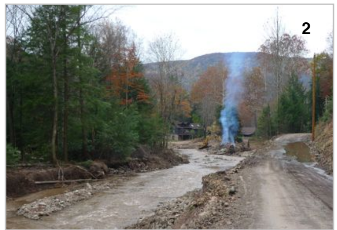
2. Snagging and burning of woody debris, gravel, realignment of channel, and installation of rock veins. (mid to late September, 2011)
