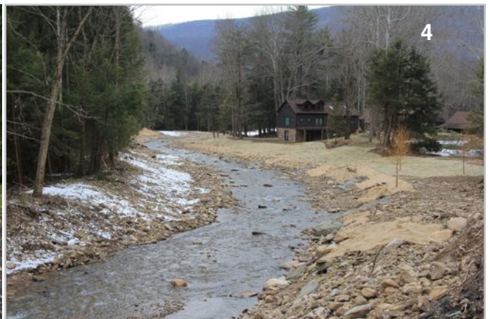
4. Reworking of channel banks, installation of rock veins on meander bend, regrading and armoring of channel banks. (October, 2011)
